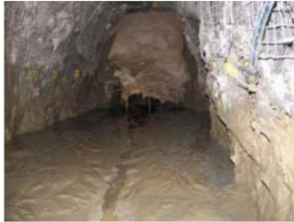
Figure 2.30 barricade failure under high hydraulic pressure (taken from Revell and Sainsbury 2007b, reprinted with permission of the Canadian Institute of Mining, Metallurgy and Petroleum)
