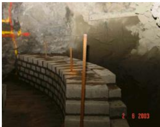
Figure 2.24 Side view of the construction of a curved barricade (Sivakugan et al. 2006, reprinted with permission of Kluwer Academic Publishers)
