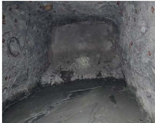
Figure 2.25 Waste rock barricade sprayed with shotcrete (Personal collection of Prof. Li Li)
