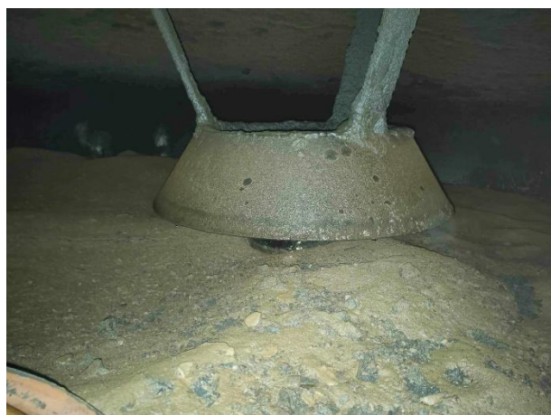
Figure B.2: Photo of the top of the cored biofilter. The media is close to the water distributor and that a thin rust-colored layer covers the top of the media.
