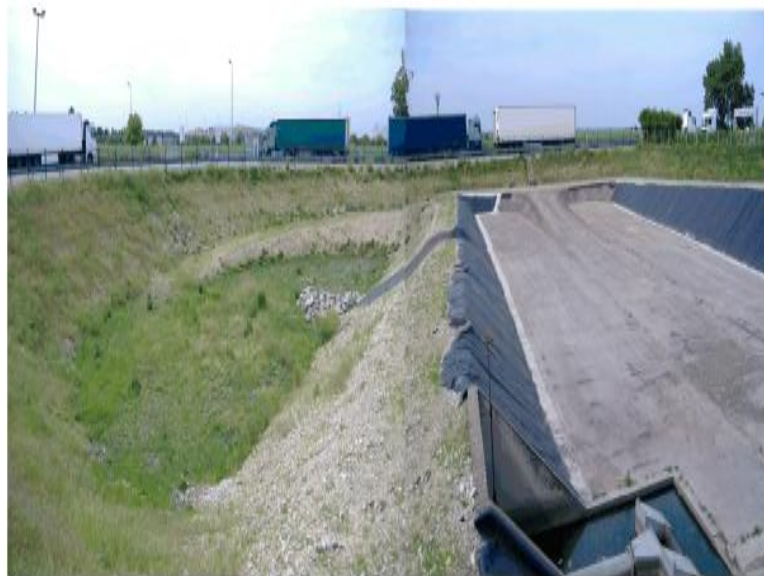
Figure 3.3 Retention/infiltration basin at the Centre routier (Moura, 2008)
