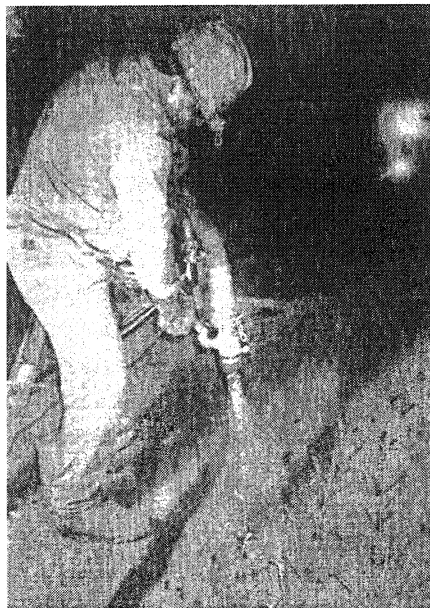
Figure 2.21 Shotcreting a refractory castable in a rotary kiln (note lack of dusting) [41].
