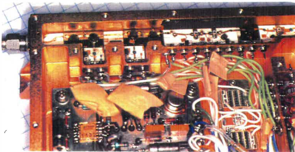
Figure 18 Detail of channel amplifier showing RF amplifier chain.
