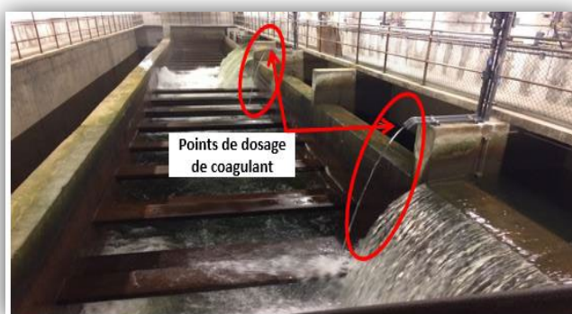
Figure 4-2. Coagulant injection point at the effluent channel of raw water pumps (see Fi. 4-3)
