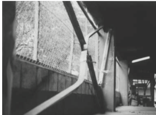
Figure 2.11 Residual inelastic buckling after a strong earthquake of a brace with low slenderness ratio. Note that the tension brace restrains laterally the compressive one. Adapted from Bruneau et al. (2011).
