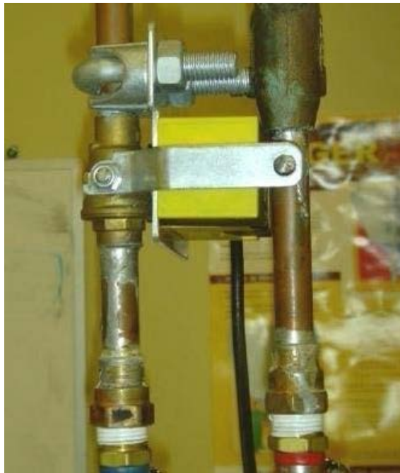
Figure 9. Inductive proximity sensor installed on the water circuit.
