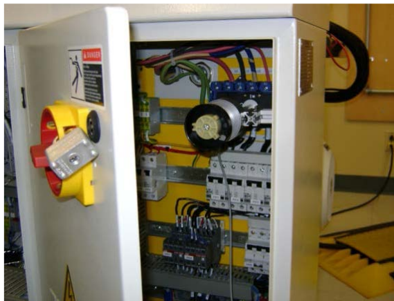
Figure 7. Rotary potentiometer installed on the electrical panel.
