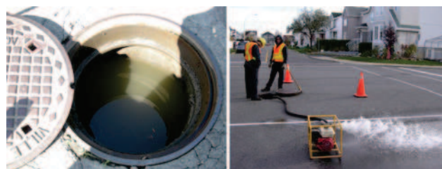
Figure 1. Flooded air-vacuum valve vault.
