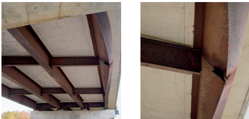
Fig. 1. Impact on girders (Photo: Edouard Berton)
