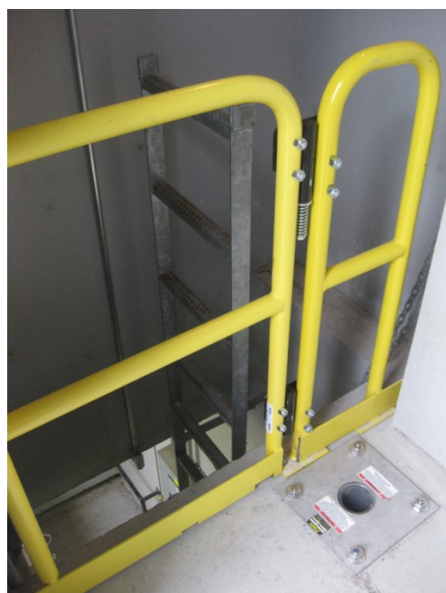
Figure 4-4 : Integration of a davit arm base, as well as a permanent ladder and guardrail
