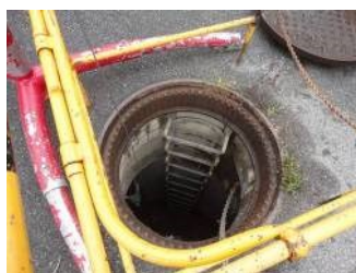
Figure 6-1 : Manhole providing access to sewer system – Scenarios #1 and 2
