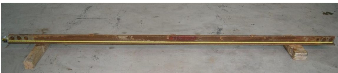
Figure 3.39: Rusted double angle brace
